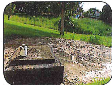
Keep septic tanks sealed.
